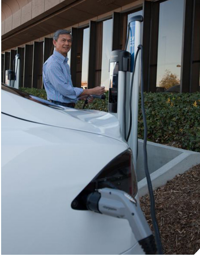
As shown, we established a corporate-level program to coordinate installation of EV stations at campuses across the company. In 2013, we added 12 EV charging stations at locations including Rancho Bernardo, California.
